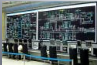
42" MPDP 13x5 / Control Center, China
