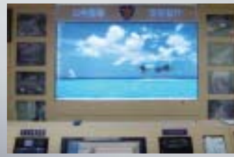
82" DID / Control Room, Korea
